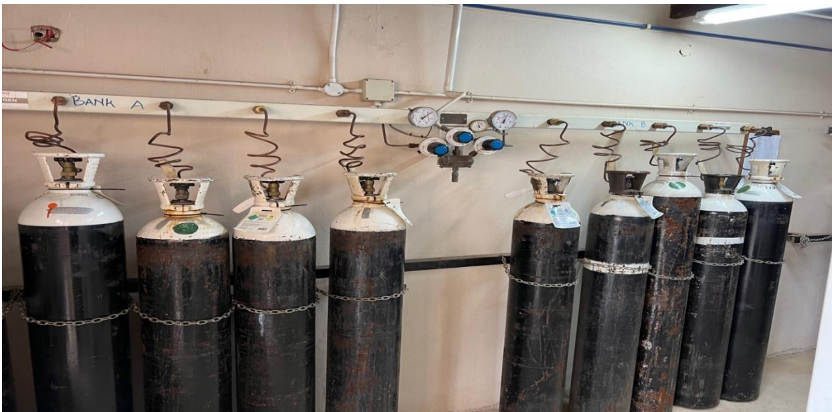
Figure 2: Existing 10-cylinder Manifold Bank
